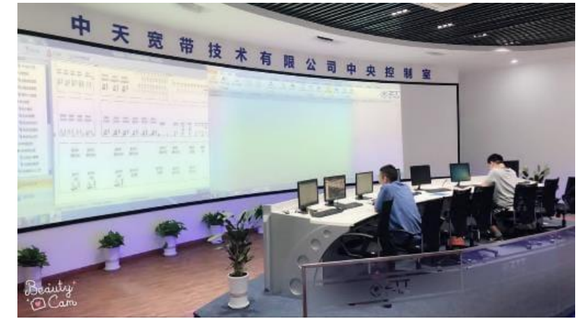
Central Control System
